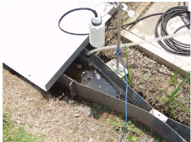
Ultrasonic modules (ISCO 710) mounted over each Parshall flume used ultrasonic reflection to measure water levels.
