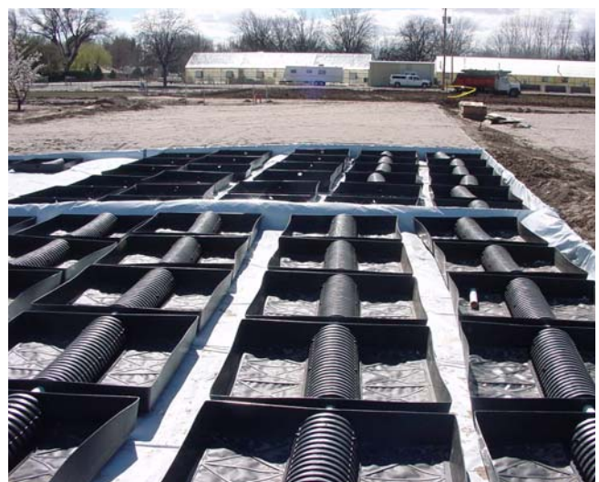
The patented subirrigation system ECS is placed at a depth of 30 cm. Slitted pipes that achieve irrigation and drainage through the same pipe system are positioned centrally inside PVC trays that measure 1.5 m x 1.5 m and are surrounded by 13 cm high sidewalls.
