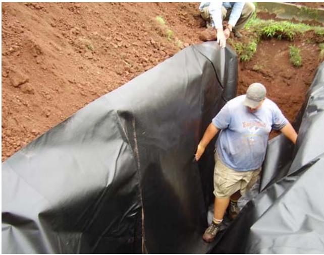
Figure 3. Each VFS in the run-on plot was 0.9 m x 4.6 m x 1.8 m, lined with an impermeable 36-mil polypropylene liner.
