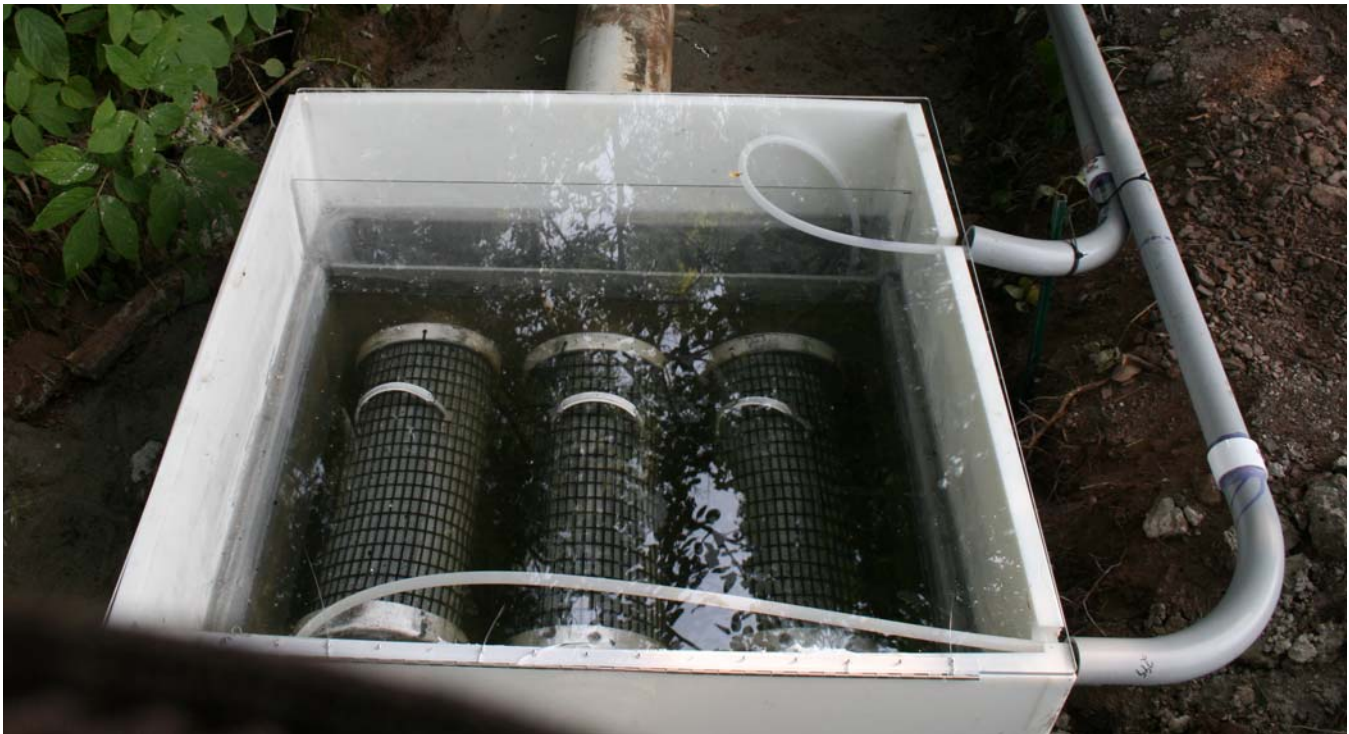
The filter system consisted of three replaceable cartridges, each approximately 600 mm long x 200 mm diameter filled with 0.015 m 3 of granular media, in a fiberglass test structure .
